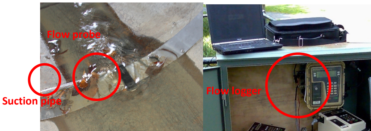
Figure 9. Typical installation of the flow sensor (left) and the above ground logger (right) installed at the Hedgeley Dene and Nunawading sites.
