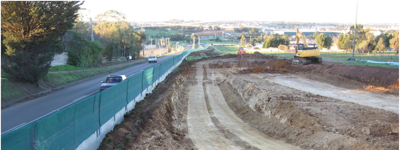
Figure 8: Screening fences providing wind suppression for a site Source Fulton Hogan
