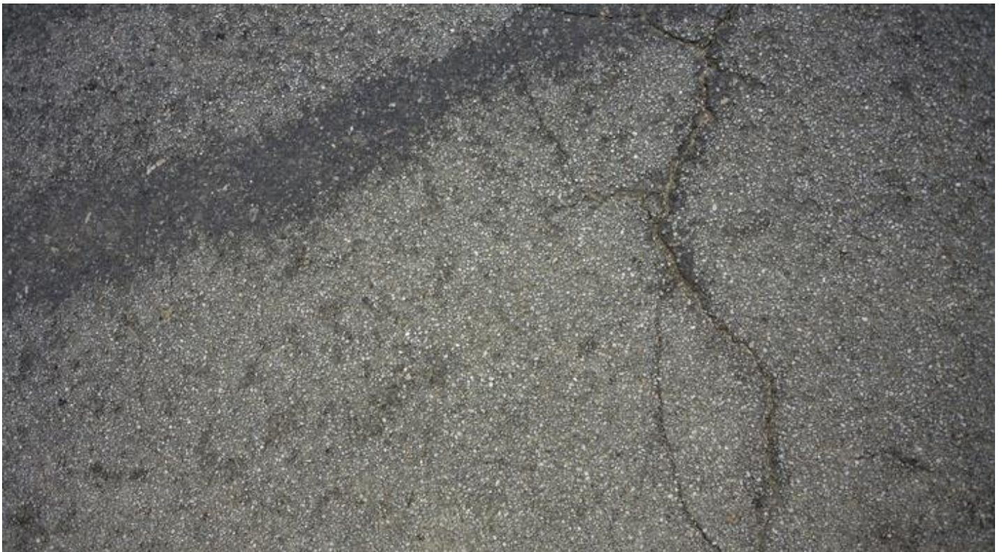
Figure 9: Cracks in surface allows runoff to leach solid materials into underlying soils Source: iStock
