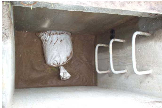
Photo 31: A Sediment Control?
