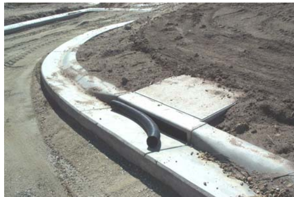
Photo 25: Agricultural Pipe Ineffectively Utilised for Kerb Inlet Protection
