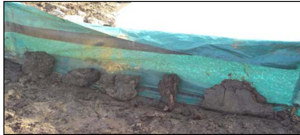
Photo 14: Sediment Fence with Inadequate Backfill
