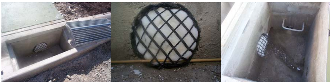
Photo 30: Silt Filtering Bung (courtesy of Statewide River and Stream Management)
