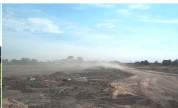
Photo 2: Dust Generation on Completely Stripped Site
