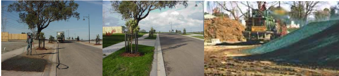
Photo 3: Hydromulching (a and b) Application for Subdivision Post Works Stabilisation (c) Application to Stockpile (courtesy of Aquaseeding)
