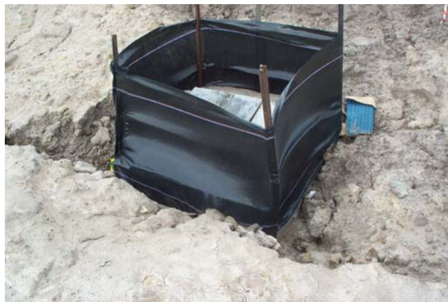
Photo 29: Erosion Under Silt Fence Pit Protection
