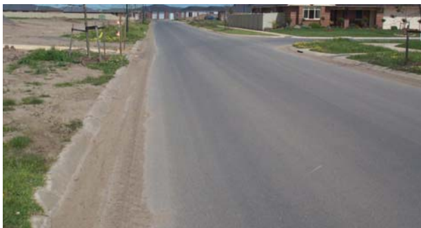
Photo 36: Sediment Left on Kerb and Gutter After Street Sweeping
