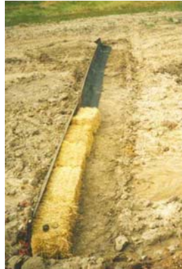
Photo 16: Straw Bale/ Silt Fence Sediment Control During Incorrect Installation
